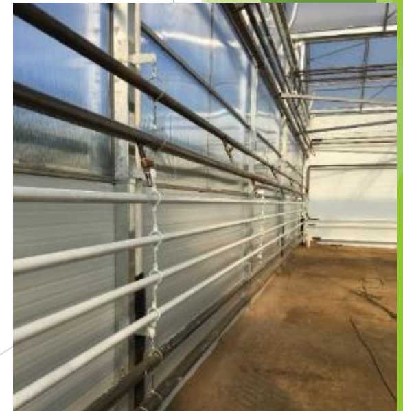
Pipes around perimeter
