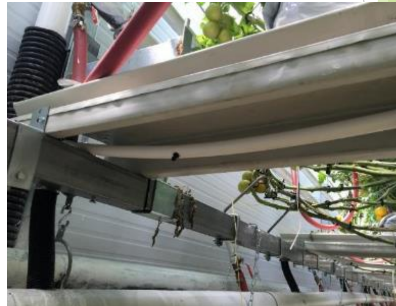
CO 2 distribution via rigid pipe
