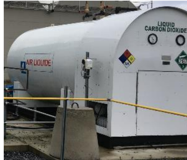
Liquid CO 2 tank
