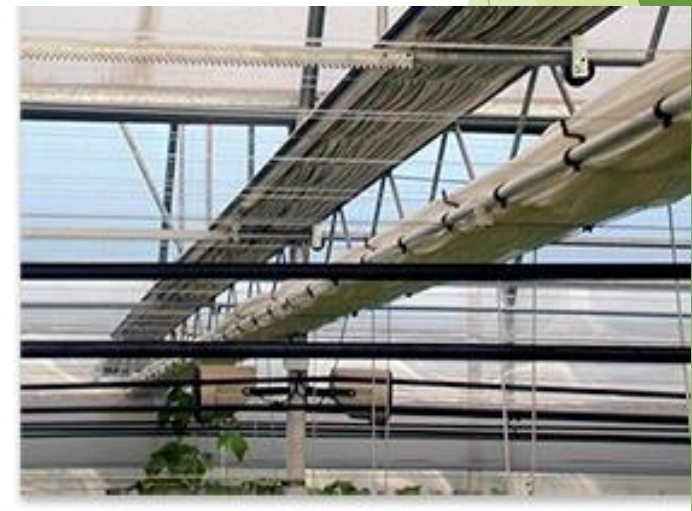
Double-layer screens on roof
