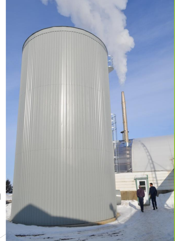
250,000-L thermal energy storage tank
