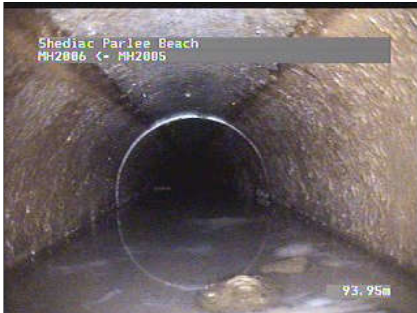
Photo: 4_4_31_A.JPG, VCR No.: 2 21.89m, Deposits Settled Fine, 10 %of cross sectional area, from 05 to 07 o'clock, , within 212mm of joint: NO
