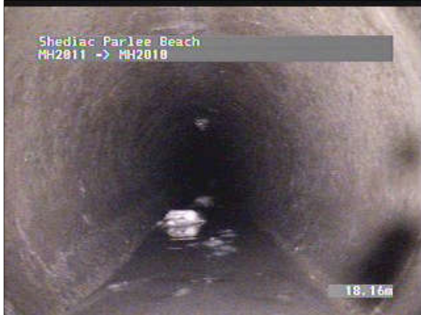
Photo: 11_11_84_A.JPG, VCR No.: 2 17.25m, Deposits Settled Fine, 10 %of cross sectional area, from 05 to 07 o'clock, , within 200mm of joint: NO, Start
