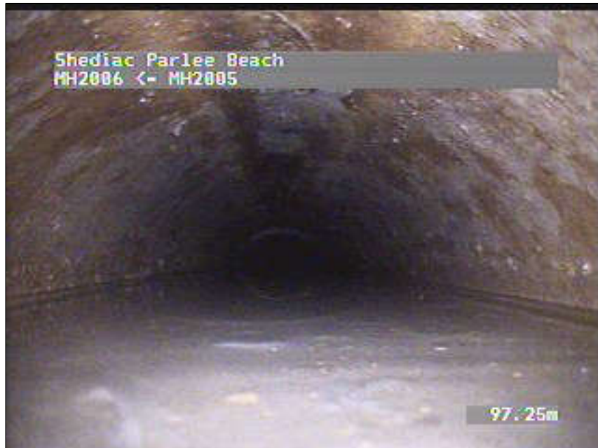
Photo: 4_4_33_A.JPG, VCR No.: 2 16m, Deposits Settled Fine, 25 %of cross sectional area, from 04 to 08 o'clock, , within 212mm of joint: NO
