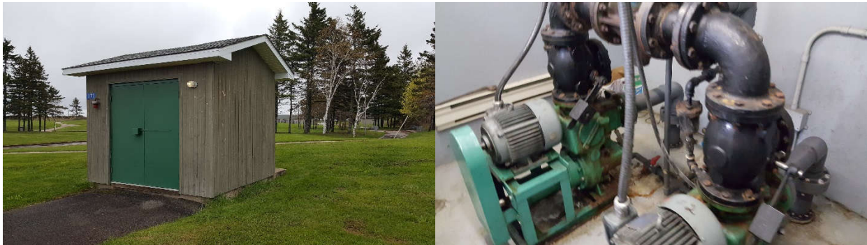
Figure 2-1 Existing Parlee Beach Lift Station
