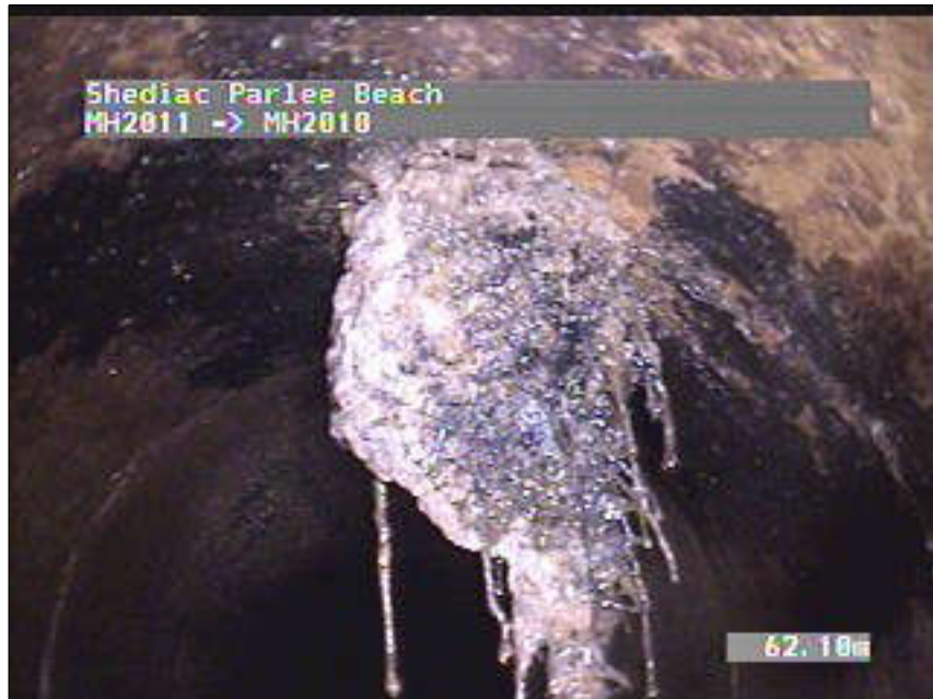
Photo: 11_11_86_A.JPG, VCR No.: 2 62.1m, Roots Medium Joint, from 12 to 01 o'clock, 15 %, within 200mm of joint: YESR
