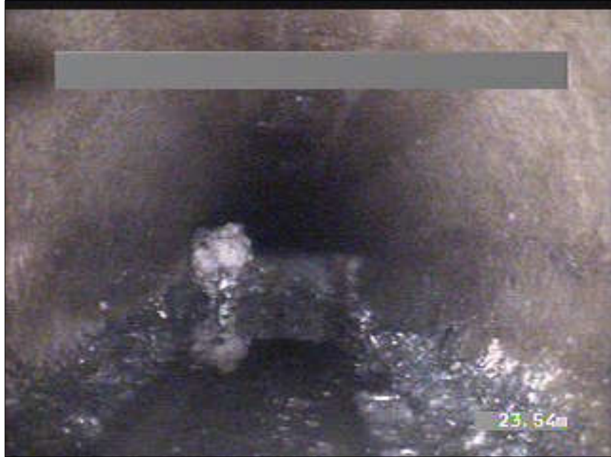
Photo: 9_9_73_A.JPG, VCR No.: 2 92.38m, Deposits Settled Fine, 15 %of cross sectional area, from 05 to 07 o'clock, , within 212mm of joint: NO, Start
