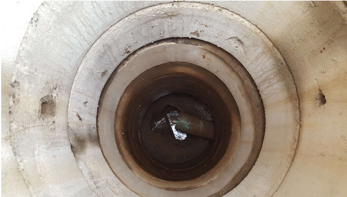
Figure 2-5 Typical Manhole at Dunes (MH2008)
