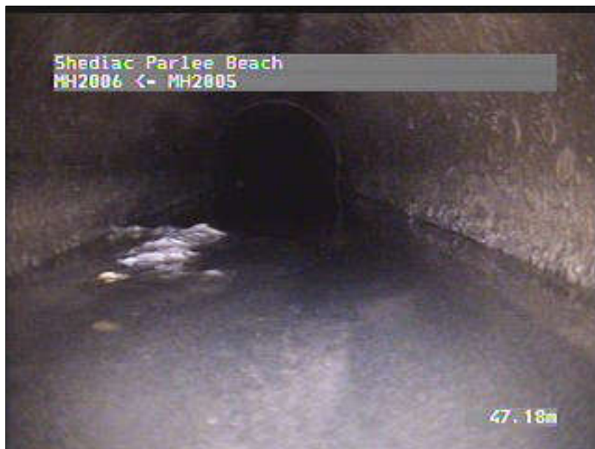
Photo: 4_4_28_A.JPG, VCR No.: 2 65.92m, Deposits Settled Fine, 15 %of cross sectional area, from 05 to 07 o'clock, , within 212mm of joint: YES
