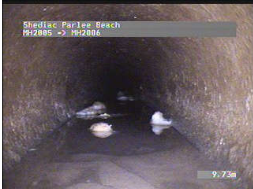
Photo: 5_5_37_A.JPG, VCR No.: 2 9.73m, Deposits Settled Fine, 15 %of cross sectional area, from 05 to 07 o'clock, , within 200mm of joint: NO, Start
