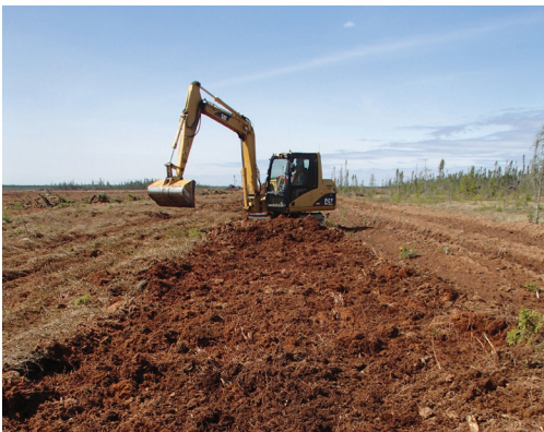
Figure 3. Collecting and picking up plant material with an excavator with wide bucket.
