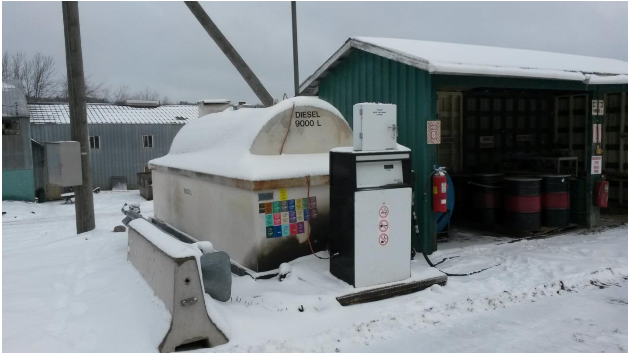
Photo 7. Petroleum Above-Ground Storage Tank (AST)
