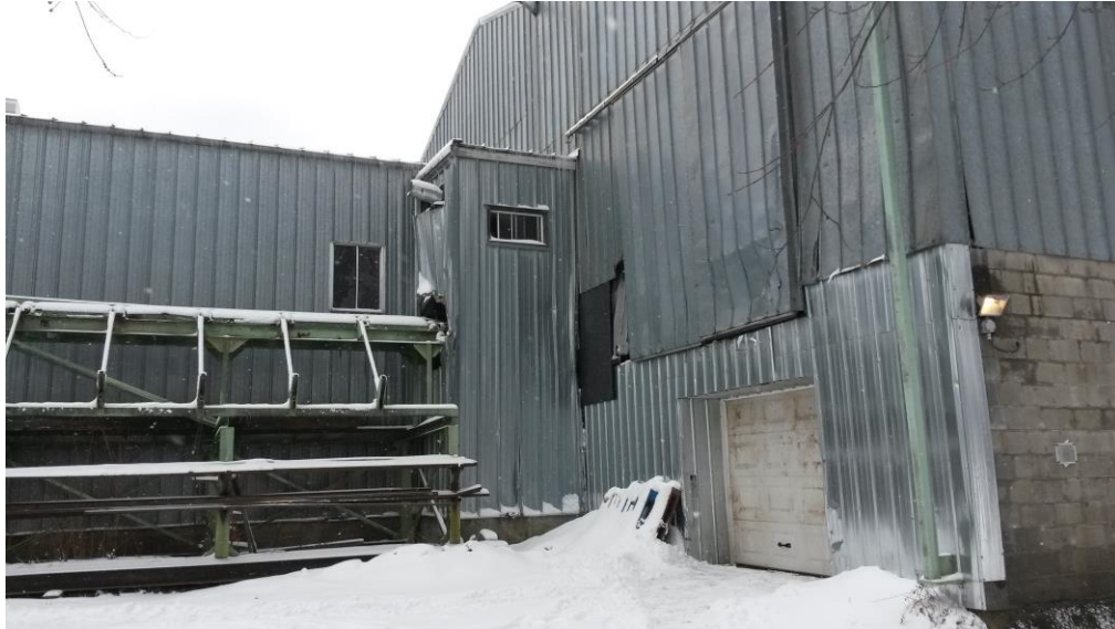
Photo 3: Exterior of sawmill showing condition of metal siding.
