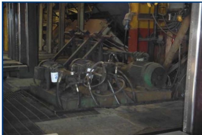
Figure 9. View of the hydraulic machinery at the subject site at 30 Progressive Drive, St. Stephen, NB. Photograph taken 26 November 2012.
