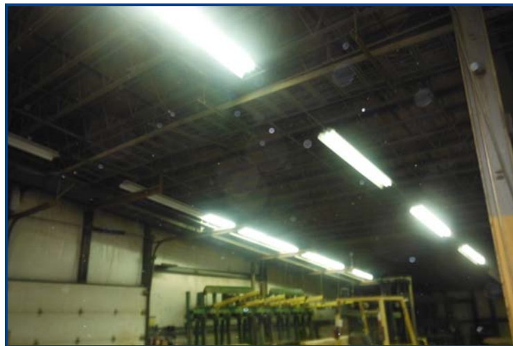
Figure 8. View of some light fixtures that may contain PCB light ballasts at 30 Progressive Drive, St. Stephen, NB. Photograph taken 26 November 2012.
