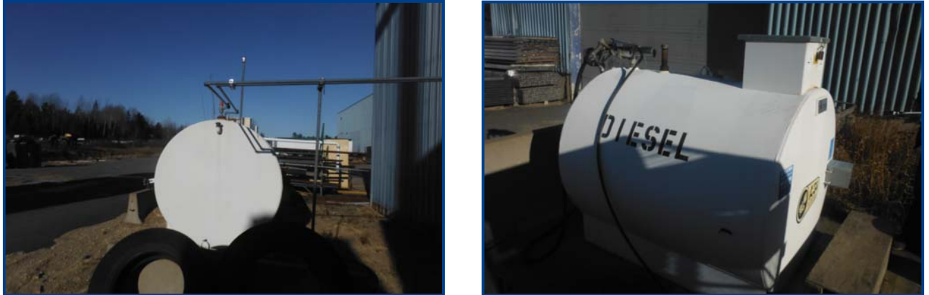
Figure 6. View of the 9092 L AST (left) and the 1980 L AST (right) located at 30 Progress Drive, St. Stephen, NB. Photograph taken 26 November 2012.
