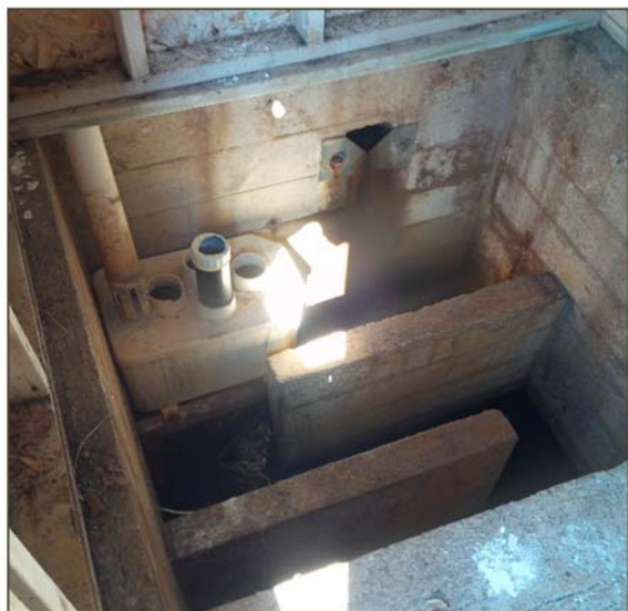
Chlorine tablet feeder
