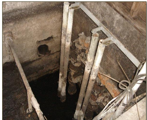
Main plant pump station
