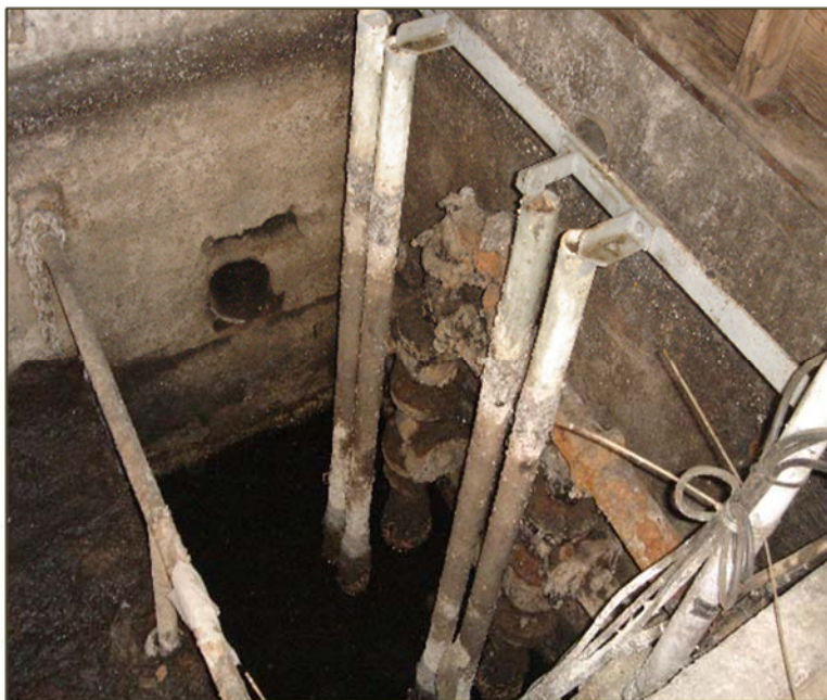
Main plant pump station
