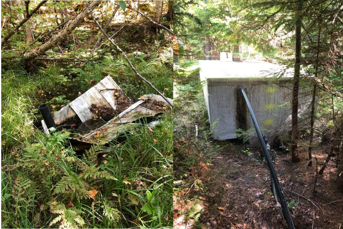
(a) Spring water intake
