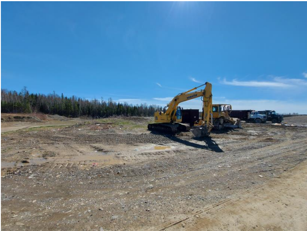
Photo 2. Equipment parking area to the south of the capped C & D cells.
