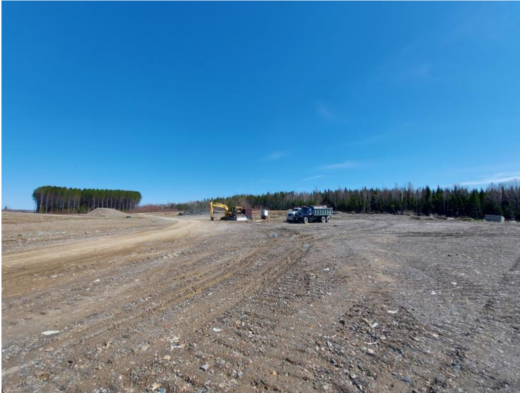
Photo 3. View from the western edge of the capped C & D cell, facing east across site towards entrance.
