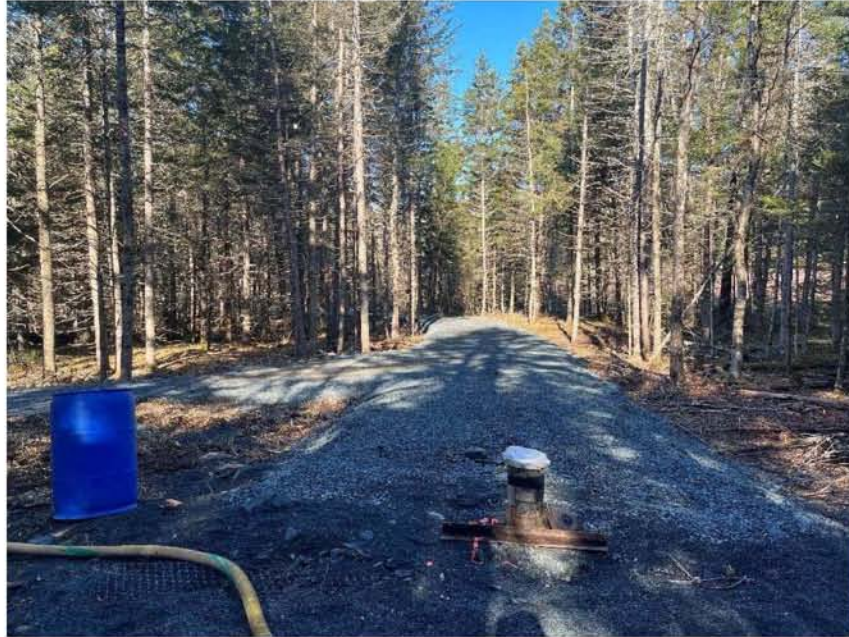
Figure 2 - Well 12, looking towards Well 10
