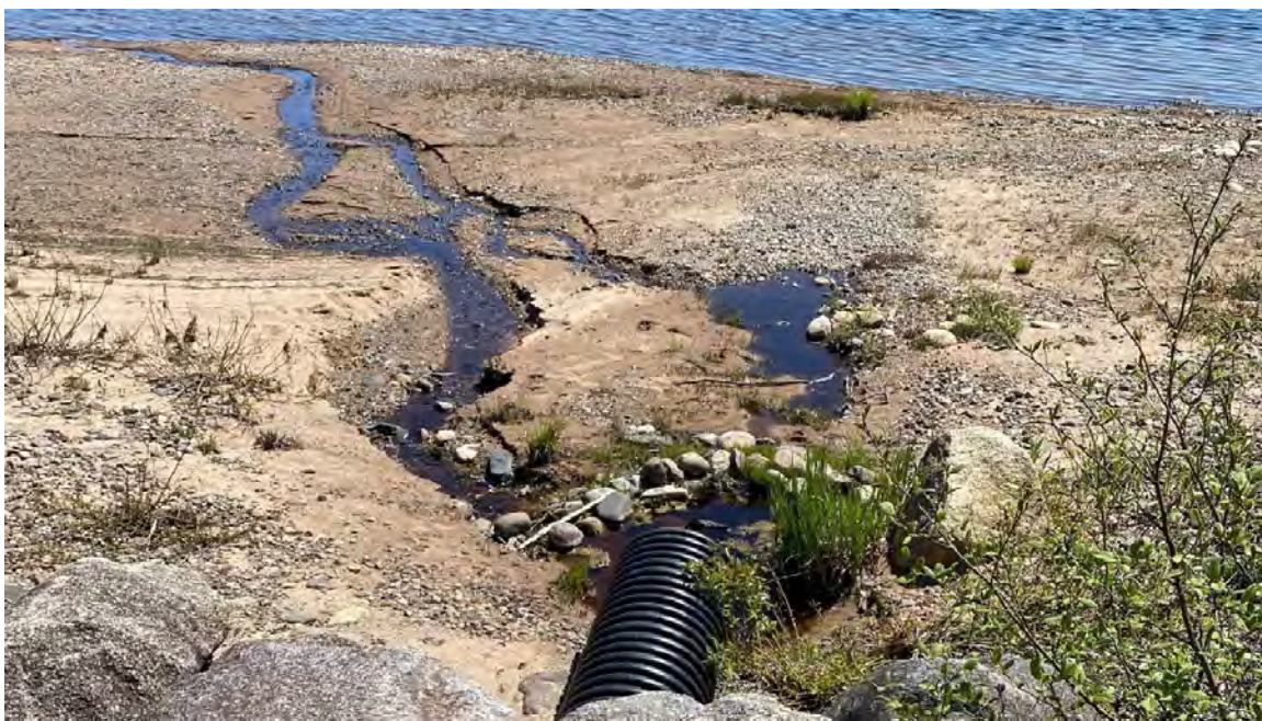
Figure 9. Photograph taken on 25 May 2022 showing the unnamed watercourse flowing from PID 15171788 under Maxwell Road in Canal, New Brunswick to the shoreline of Lake Utopia.
