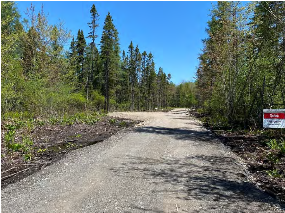
Figure 6. Photograph taken on 25 May 2022 showing the newly constructed gravel roadway extending from Wright Lane to the proposed lots on PID 15171788 in Canal, New Brunswick.
