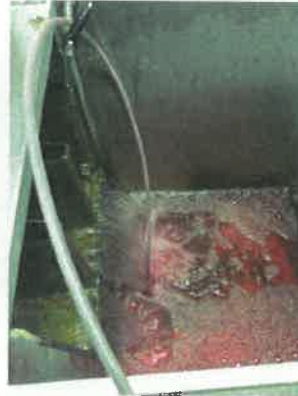
Dye injection at outlet of UV system
