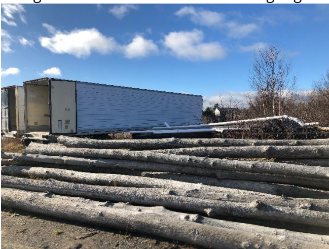
Photo 5: Wood poles and pipes and other material stored in the laydown area of Section A.
