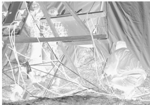
Plate 4.14: The electrical subsystem.
